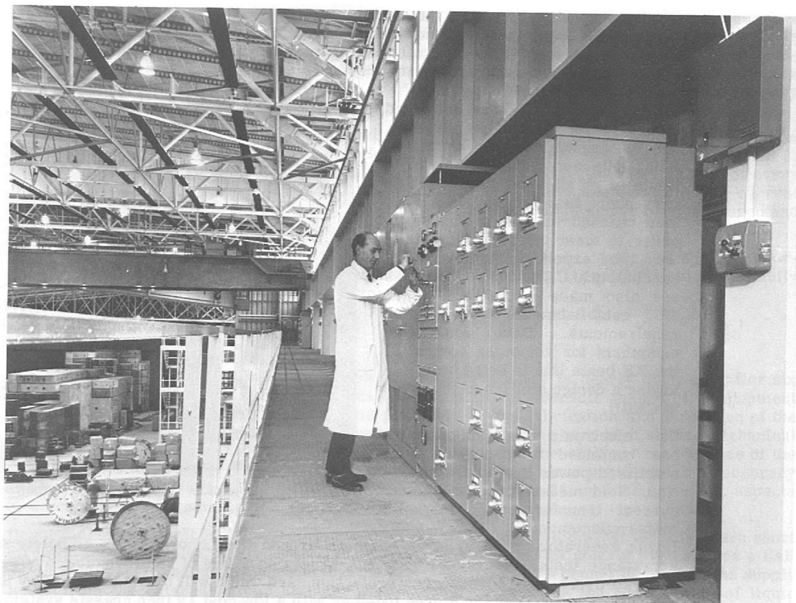
Figure 84. One of the 2.5 MW packaged substations in Hall 3.
